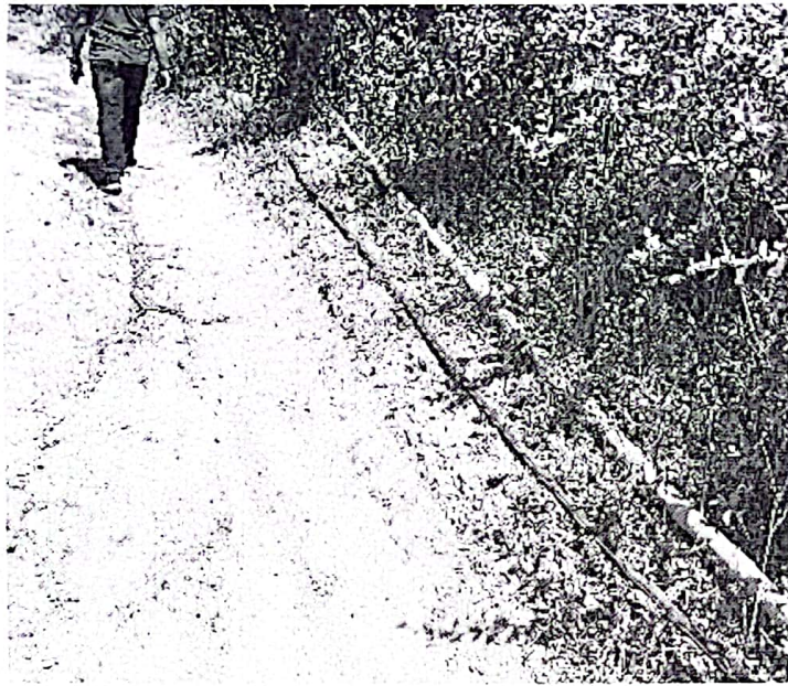
Steel pipe used for drinking water supply that needs relocation during road construction
